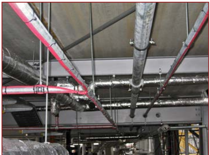
Industrial pipe tracing application.
