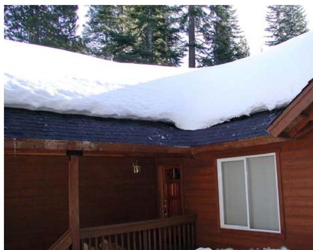
Roof deicing system heating roof edges.
