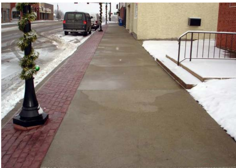
ProLine heat cable embedded in city sidewalks.
