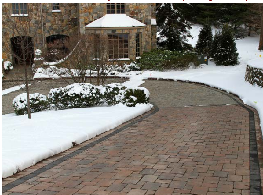
ProLine snow melting system installed in paver driveway.
