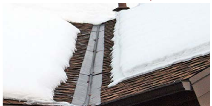
ProLine low-voltage roof deicing system heating roof valley and edges.
