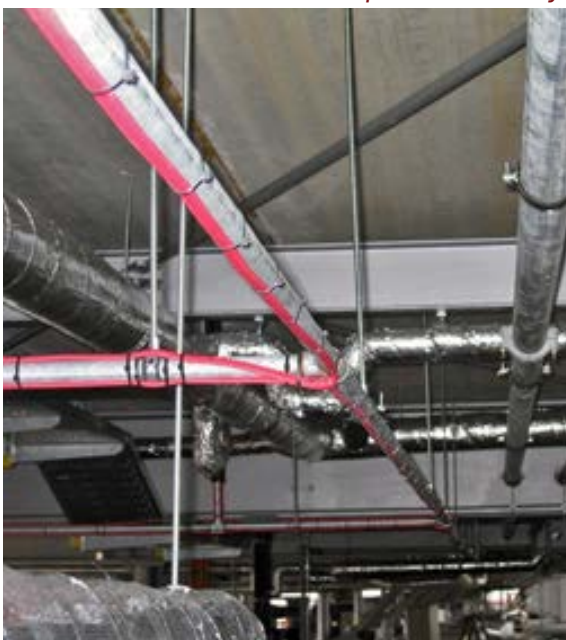
Pipe tracing system installed.
