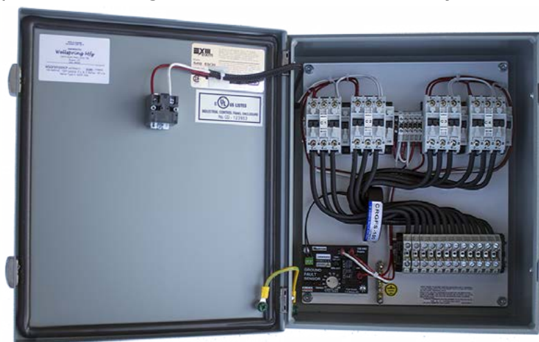
Control panel opened.
