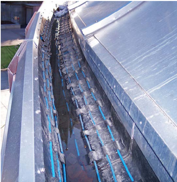
ProLine roof deicing heat cable installed in commercial gutter melt application.
